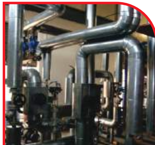
THERMAL OIL HEATER PIPING
